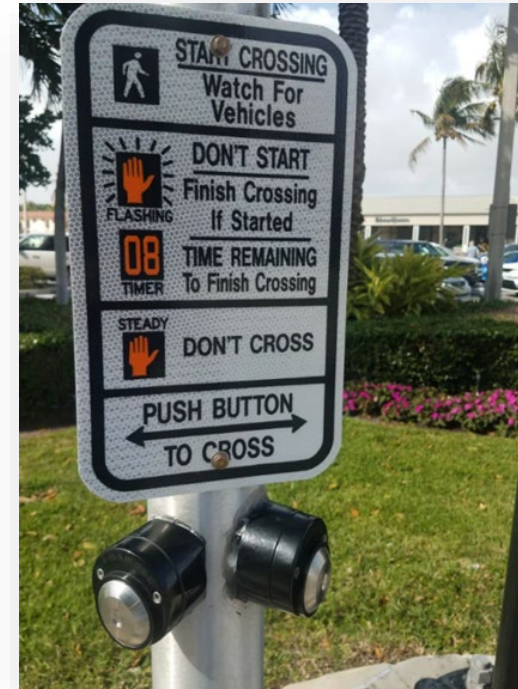
Replacement of pedestrian push-buttons and signal heads to meet Americans with Disabilities Act (ADA).
